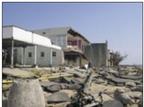
BEACH BOULEVARD IN BAY SAINT LOUIS SHOWING SOME OF THE REMAINING BUILDINGS AND WHAT USED TO BE THE ROAD BED.
