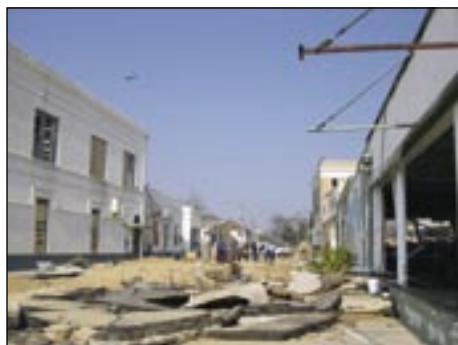
VIEW OF THE DAMAGE TO THE BUILDINGS ON MAIN STREET IN BAY ST. LOUIS
